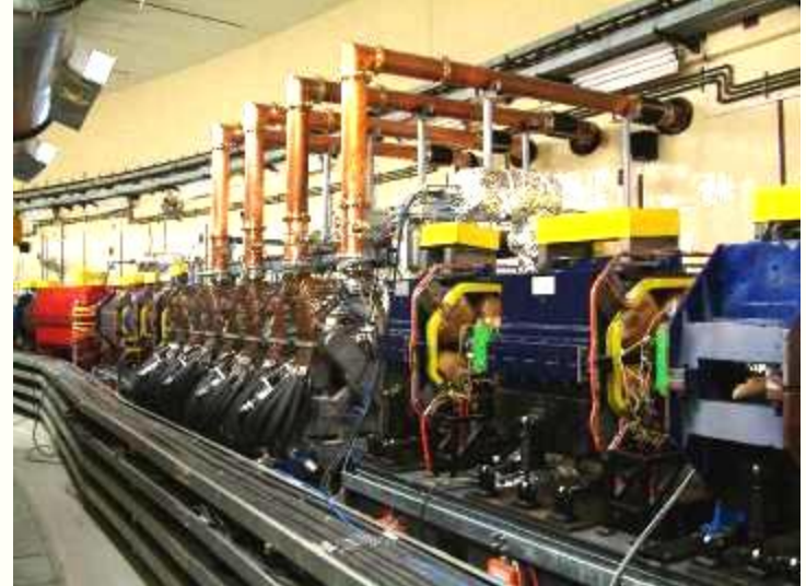
RF Cavities installed in Indus-2 Ring
