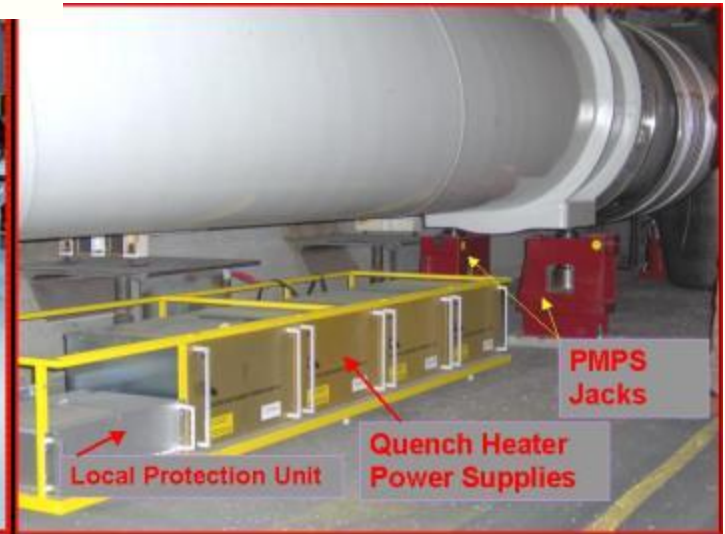
A part of DAE's contributions installed in LHC Tunnel at CERN
