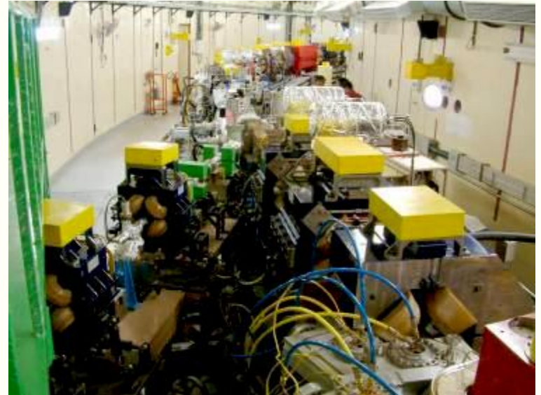
Transport Line-3 Joining on to Indus-2
